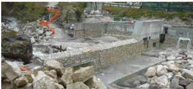
Figure 3. A highly contested hydropower plant in the Piave River Basin, being masked by a natural stone clap.
