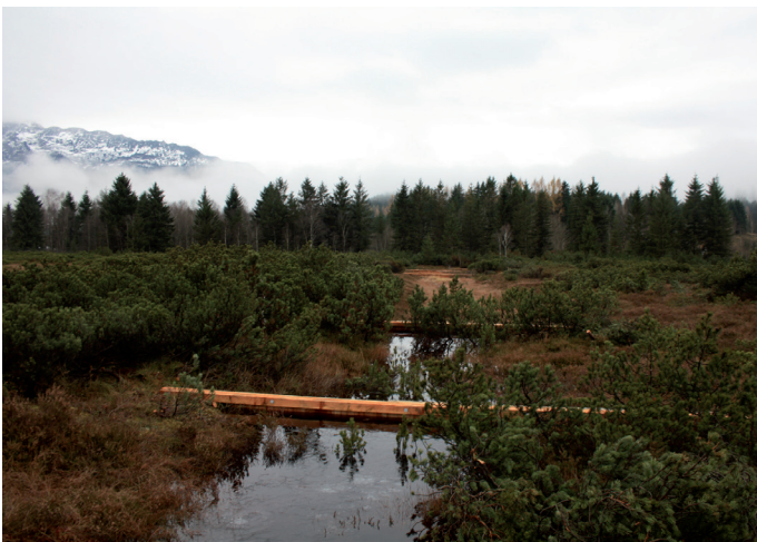
Figure 11 & 12 – Larch planks are pushed with great precision down into the ground. Once the work is done, the water accumulates and spreads into the bog area. © ÖBf-Archiv/A.-S. Pirtscher
