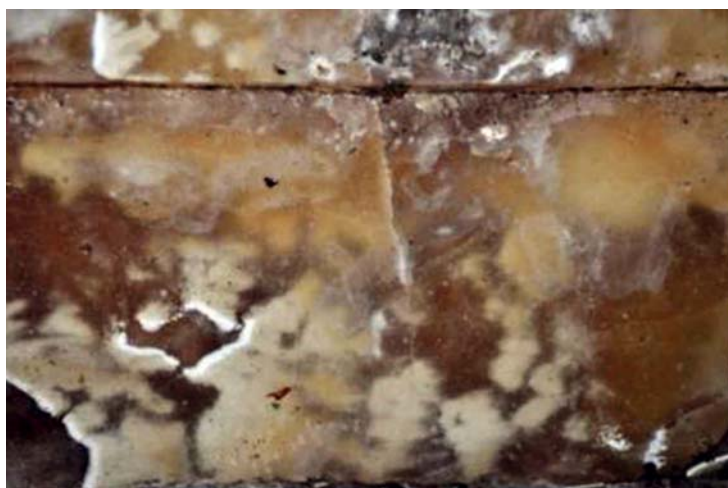
Abb. 6: Villa A (Oplontis), Room 14 alabaster threshold
