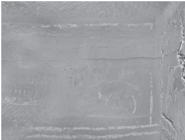
Fig. 19 El-Sheikh Fadl – Umm Raqaba. Decorated wall section of the chapel of tomb A2 T1 (Panel 1) (Photo: E.G. Hammerschmid)
